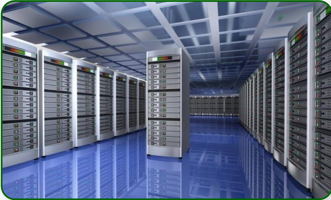
High Availability Data Center Infrastructure
